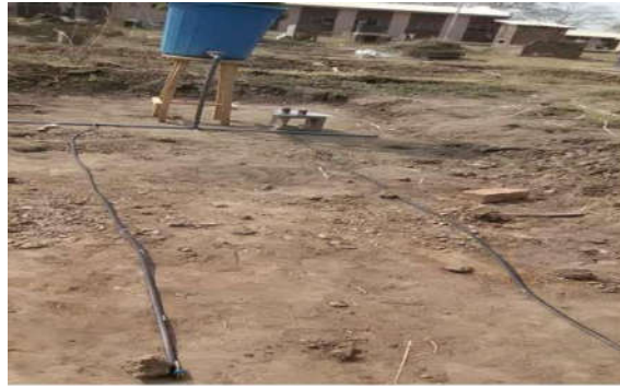
Plate 2: Irrigation line setup
