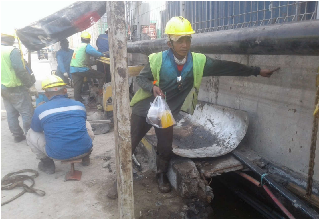
Photo 2. A worker pointed to the rob height dated May 23, 2022 on a concrete wall in the Semarang Port Area (Personal documentation July 28, 2022).
